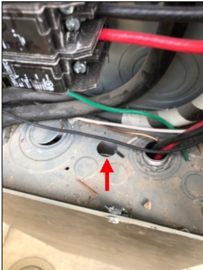
Exposed knock at base of the electrical panel (4), safety hazard recommend repair.
