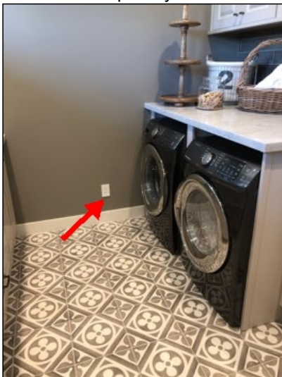
Electrical outlet at laundry room main floor north wall is non functional (2), Recommend further review and repair by licensed contractor.
