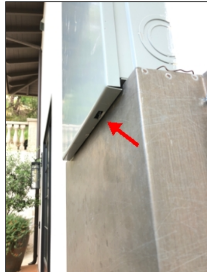
Main electrical panel cover does not latch properly due to metal panel directly underneath *, recommend repair.
