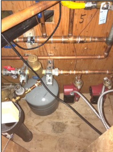
Tankless water heater plumbing appears serviceable.
