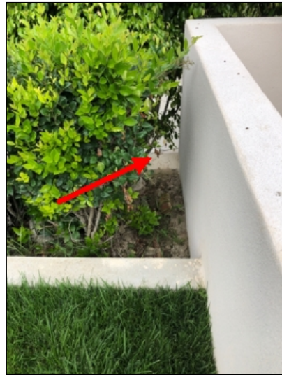
Front patio/lawn area does not have a railing installed (4), safety hazard. Small child may fall. Recommend repair as a safety upgrade.
