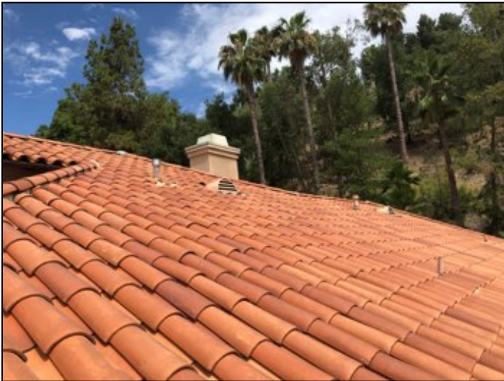
Main roof is clay tile, the majority of roof appears serviceable with few broken tiles. Recommend having broken roof tiles repaired as required to prevent moisture intrusion.
