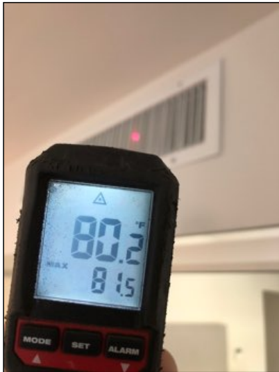
HVAC unit (B) on heating mode temperature is 80°F, appears serviceable.
