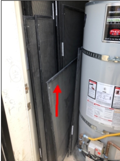
Property screens stored in water heater closet
