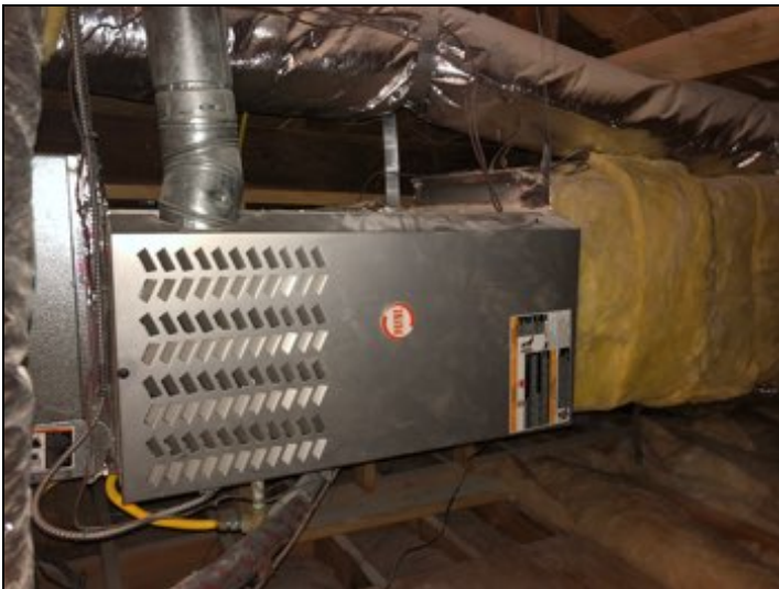
HVAC unit services Kitchen located in attic. 88,000 Ton
