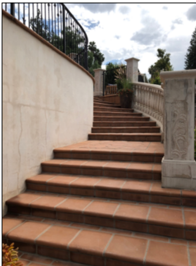
Front entrance railing not installed a base of stairs located at front *(4), recommend installing as required.
