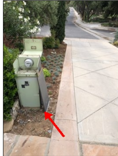
Main electrical panel container located at driveway does not have a protective bollard to prevent damage from a automobile strike *, recommend installing as an upgrade.
