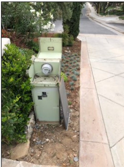
Main electrical panel breaker/meter located at driveway.
