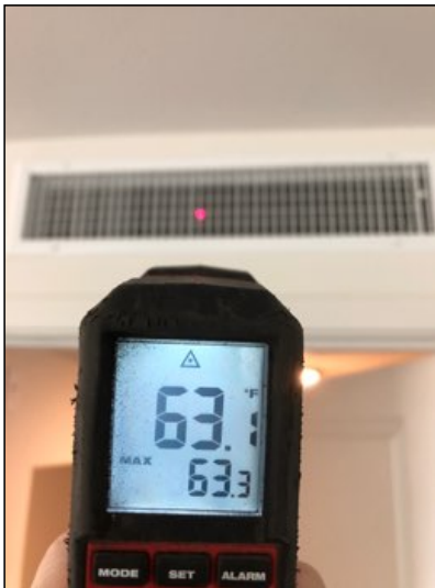
Unit (E) temperature on cooling mode is 63°F, appears serviceable. Services third floor.
