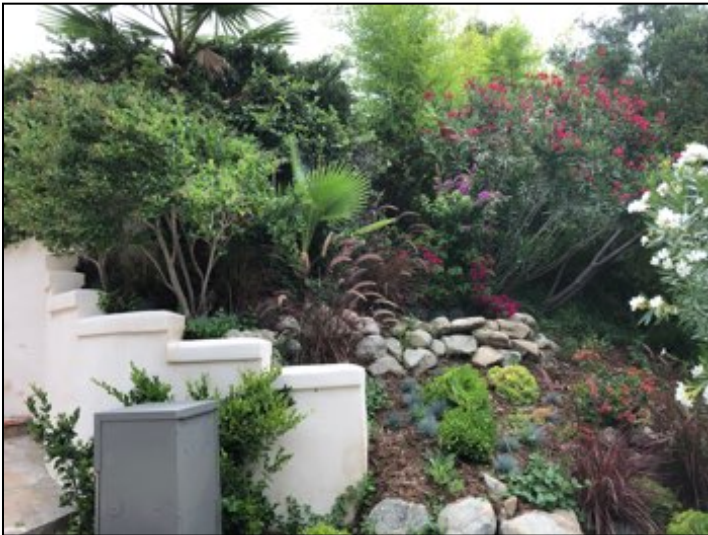
Retaining walls located on: South side is masonry block wall, appears serviceable.
