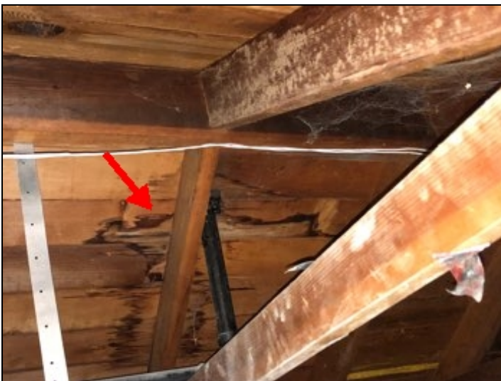
Moisture stains visible in attic space roof framing at various areas *, inspector could not determine if leaks are active *, inspection is limited (2). Recommend having all roof tiles that are broken and flashing mentioned on roofing section repaired along with having a licensed roofing contractor further review roof.
