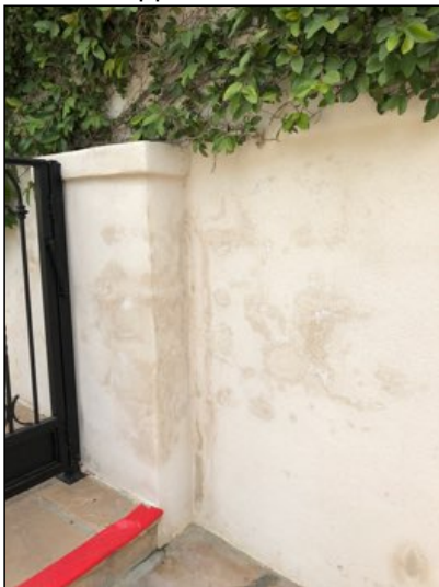
Retaining walls located on: West side is masonry block wall, appears serviceable.
