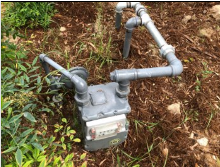
(South) Main gas supply Meter is located on south side of property. Main gas supply shut off valve installed, appears serviceable.
