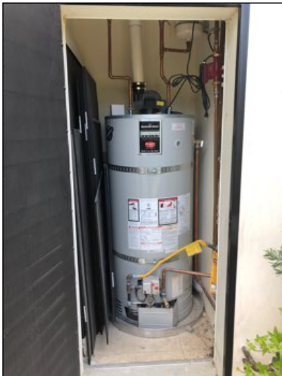
Water heater appears serviceable, see sections below for other notes and or issues with water heater.
