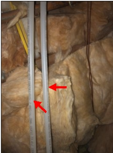
Water supply pipes are PEX (Crosslinked Polyethylene). Some name brands such as Aquapex, Zurn, and Kitec have been associated with class action law suits. Failures from pipes included: Leaching of chemicals into potable water, Pipe fitting premature corrosion causing leaks, as well as other documented issues. The brand name installed at property does not appear to be associated with failures but does not guarantee no issue or failures will ever occur with PEX piping. Inspection is limited.
