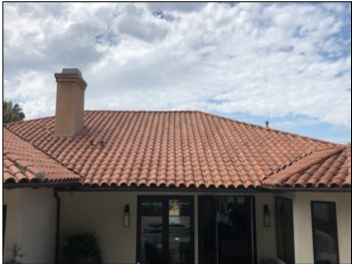
Main roof is clay tile, the majority of roof appears serviceable with few broken tiles. Recommend having broken roof tiles repaired as required to prevent moisture intrusion.
