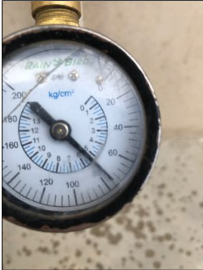
Main water supply pipe pressure is 75 psi., appears serviceable.
