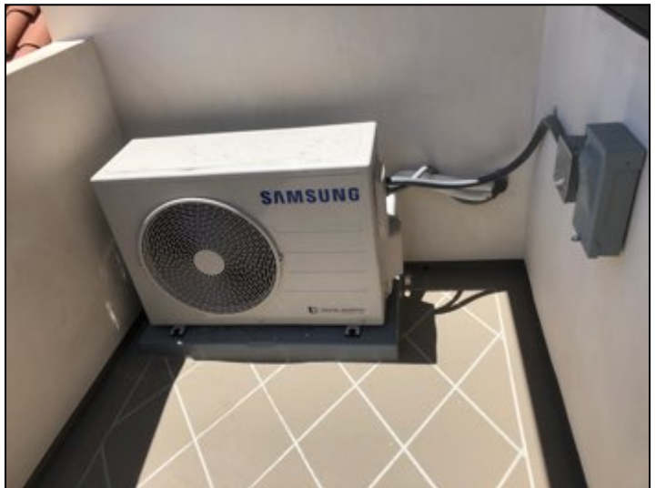
Unit (E) heat pump services third/top floor.
