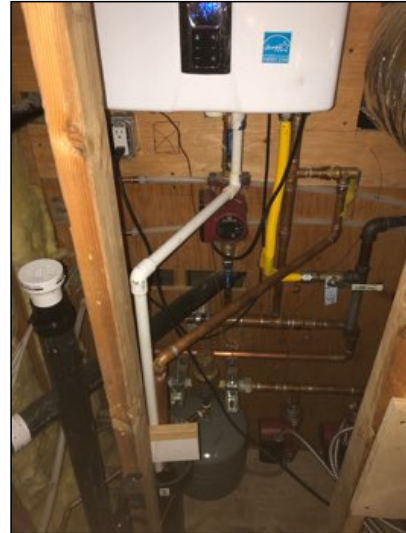
Tankless water heater located in attic does not have a water catch pan installed that will catch water in case of leak *, recommend installing as an upgrade.
