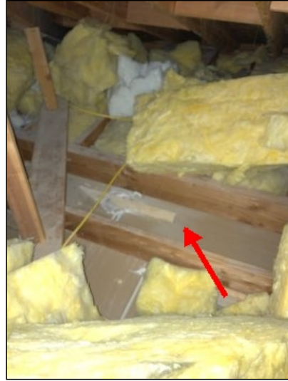
Few areas in main attic has missing/displaced insulation *. Recommend repair.
