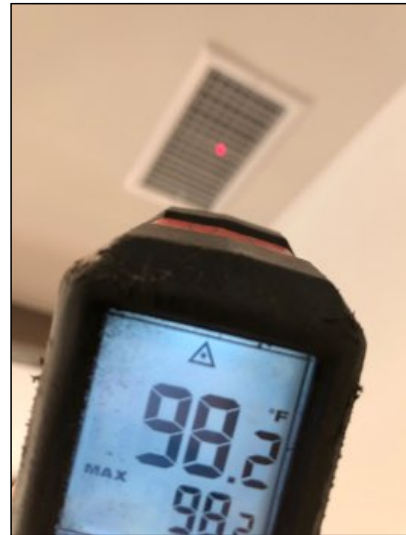
HVAC temperature on heating mode for master bedroom is 98°F, appears serviceable.
