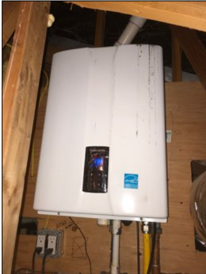
Tankless water heater installed, appears serviceable, see notes below for other issues that may be associated with Tankless water heater.
