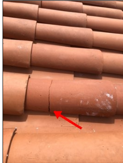
Broken clay tile at third floor visible from second floor balcony (2), recommend repair.
