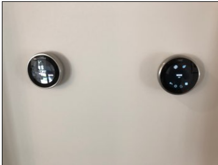
Radiant flooring thermostats located at main hallway leading into master bedroom.
