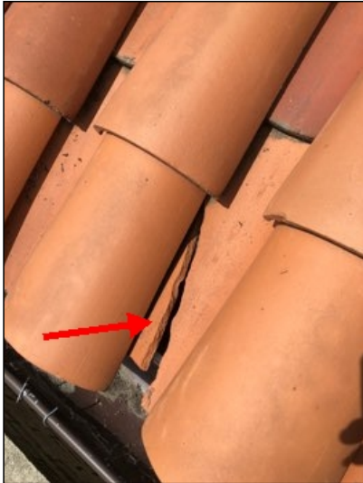
Roof clay tile is broken located on east side (2), recommend repair to prevent moisture intrusion.
