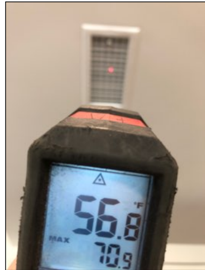
Unit (A) cooling mode temperature is 56°F, appears serviceable.
