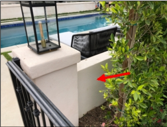
Masonry block wall located at front for pool area appears to be too short allowing small child to climb over (4), safety hazard. Recommend repair as required.
