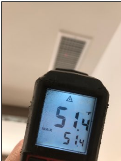
HVAC cooling mode in Master bedroom temperature is 51°F, appears serviceable.
