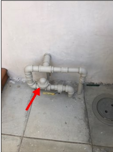
Automatic gas seismic shut off valve installed at main gas supply pipe, appears serviceable.
