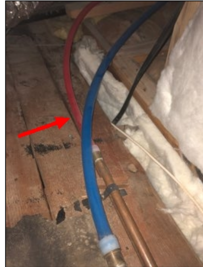
Water supply pipes are PEX (Crosslinked Polyethylene). Some name brands such as Aquapex, Zurn, and Kitec have been associated with class action law suits. Failures from pipes included: Leaching of chemicals into potable water, Pipe fitting premature corrosion causing leaks, as well as other documented issues. The brand name installed at property does not appear to be associated with failures but does not guarantee no issue or failures will ever occur with PEX piping. Inspection is limited.
