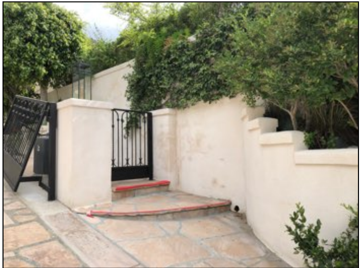
Retaining walls located on: West side is masonry block wall, appears serviceable.
