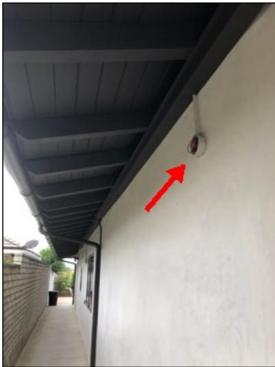
Exterior west side light fixture is missing with exposed live electrical conductors (4)(2), safety hazard. Recommend further review and repair by licensed contractor.
