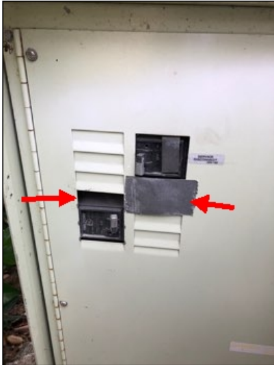
Main electrical panel has exposed knock outs at missing breakers (4), safety hazard recommend repair. Improper tape was installed to cover exposed knock outs.
