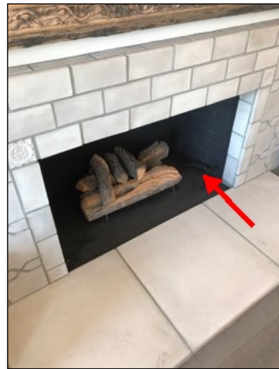
Fireplace does not have a spark screen installed as required (4), safety hazard.
