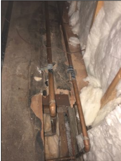
Water supply pipes that are visible are copper, appears serviceable. See notes below for other issues that may be present.
