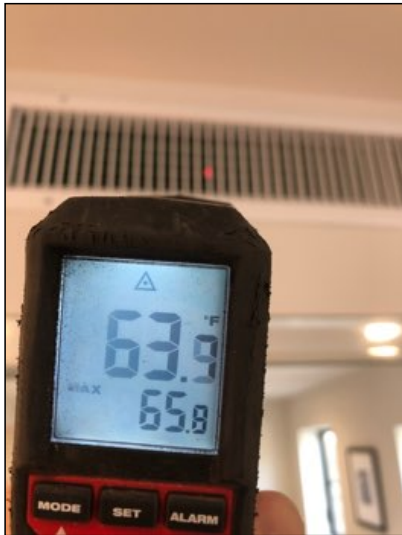
Unit (B) on cooling mode temperature is 68°F, appears serviceable.
