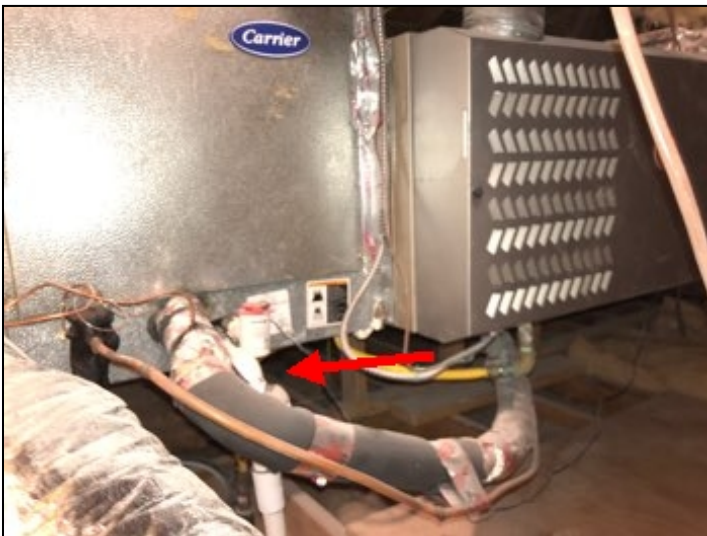
Cooling coil at furnace located in attic did not have a secondary catch pan installed, recommend installing catch pan to catch condensation from cooling coil as required *. Secondary catch pans are recommended to insure excess condensation does not cause moisture damage. Secondary catch pans required at all HVAC unit in attic.
