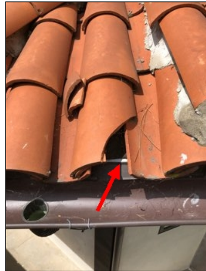
Roof clay tile is broken located on NE corner (2), recommend repair to prevent moisture intrusion.
