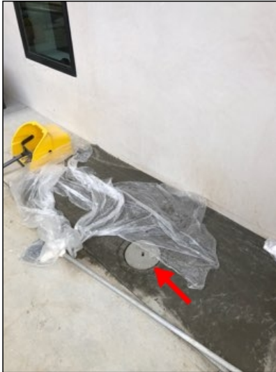
(clean out W) Waste clean out pipe located west side of property.
