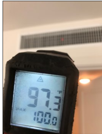
Unit (E) temperature on heating mode is 97°F, appears serviceable.
