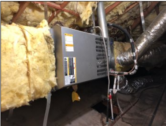
HVAC furnace services Dining room located attic over stairwell. 110,000 TON
