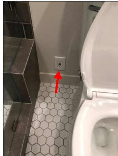
Bathroom (E) GFCI electrical outlet did not reset when tested *, inspector could not locate other GFCI that will reset and or outlet is miss wired *.
