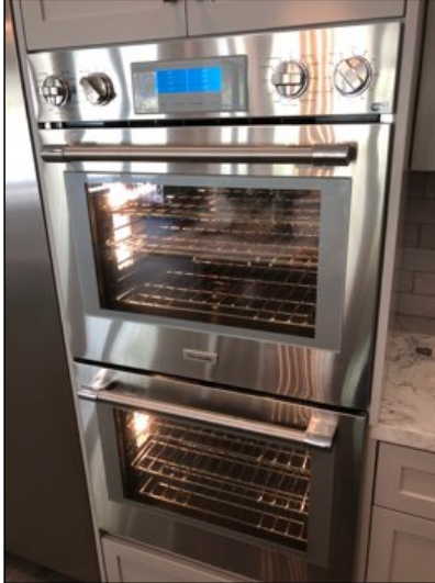
Oven(s) are/is electric, appears serviceable.
