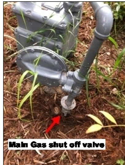
(South) Main gas supply Meter is located on south side of property. Main gas supply shut off valve installed, appears serviceable.
