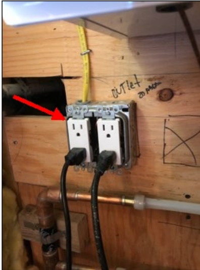
Various attic electrical light switches are missing cover plates *(4), recommend installing as required.
