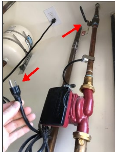
Water heater recirculation pump is not connected to electrical and water is shut off *.
