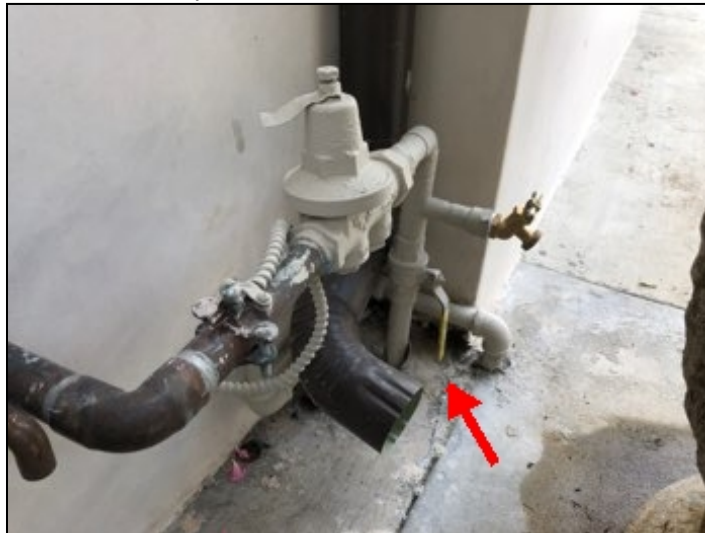
(west) Main water shut off valve installed located on west side of property, valve appears serviceable.
