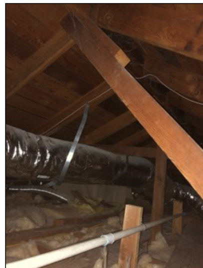
Attic structure is conventional wood framing 2x6 ceiling joist and 2x6 roof rafters, plywood roof.
