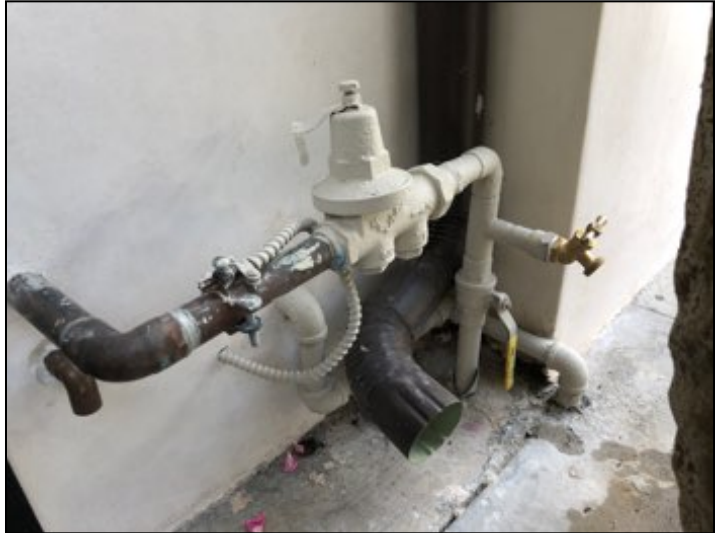
(no pressure exhaust) Main water supply pipe does not have a pressure exhaust installed as required (2), recommend installing. Recommend further review and repair by licensed plumber.
