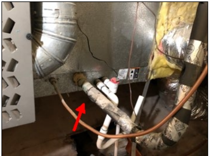
Cooling coil at furnace located in attic did not have a secondary catch pan installed, recommend installing catch pan to catch condensation from cooling coil as required *. Secondary catch pans are recommended to insure excess condensation does not cause moisture damage. Secondary catch pans required at all HVAC unit in attic.
